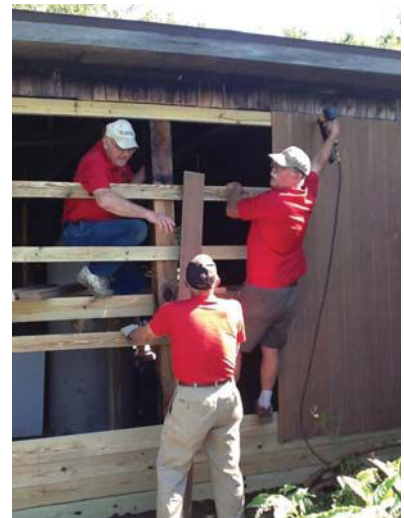
Lions (from left) Ward Holdsworth, Ken Sopher and Neil Rupe work on the storage building.
